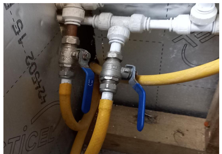
MT Area Drain Valves – Open Position
